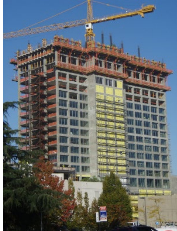
(b) High-rise moment frame-wall building in Pacific Northwest of United States. (Photograph courtesy of Cary Kopczynski)
