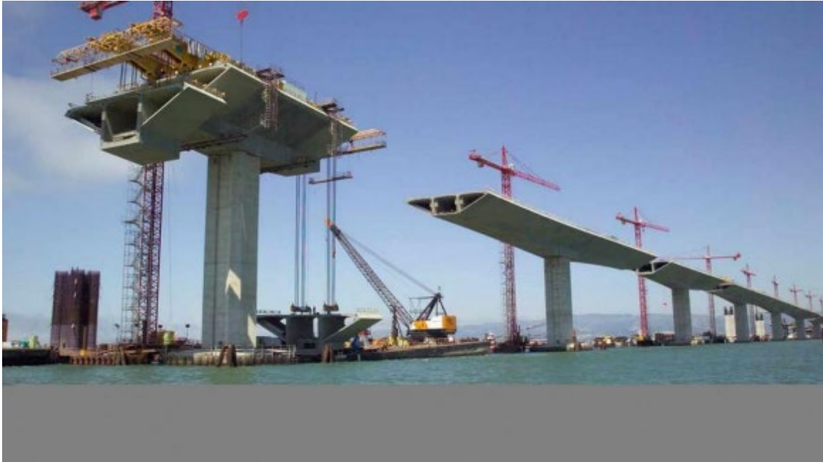
Figure 15-3 Construction of the San Francisco Oakland Bay Bridge Skyway. Note the segmental precast construction, in which precast segments are hoisted into position, then prestressed and grouted in place. ( http://www.hatchertechnical.com/ )
