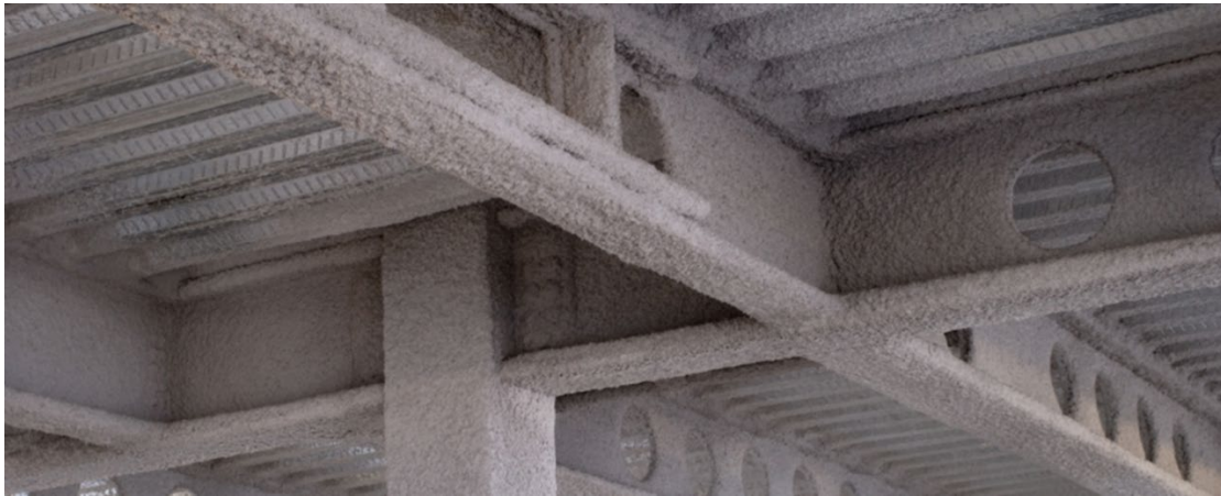
Figure 14-4 Fire protection of structural steel members. Top: Intumescent paint before and after fire exposure ( http://vmp-holding.com/ ). Bottom: Cementitious fire spray ( http://www.sharpfibre.com/ ).
