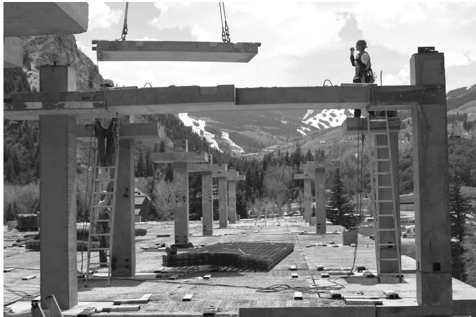
FIGURE 19.18 Precast slab element with precast columns, beams, and lateral framing. (Photograph by Charles W. Dolan.)
