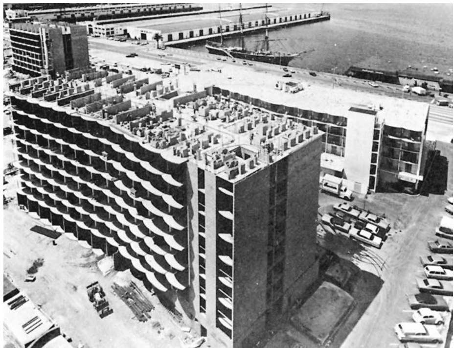
FIGURE 17. Construction of a high-rise motel using reinforced concrete masonry walls. (Courtesy of Portland Cement Association)
