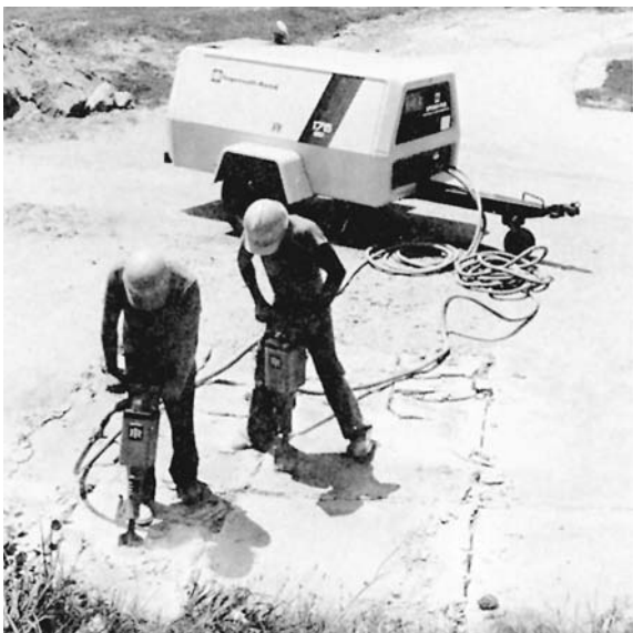
FIGURE 2. Small portable air compressor powering pneumatic tools. (Courtesy of Ingersoll-Rand Company)
