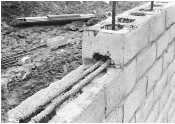
FIGURE 18. Placement of reinforcing steel in reinforced concrete masonry wall. (Courtesy of Portland Cement Association)
