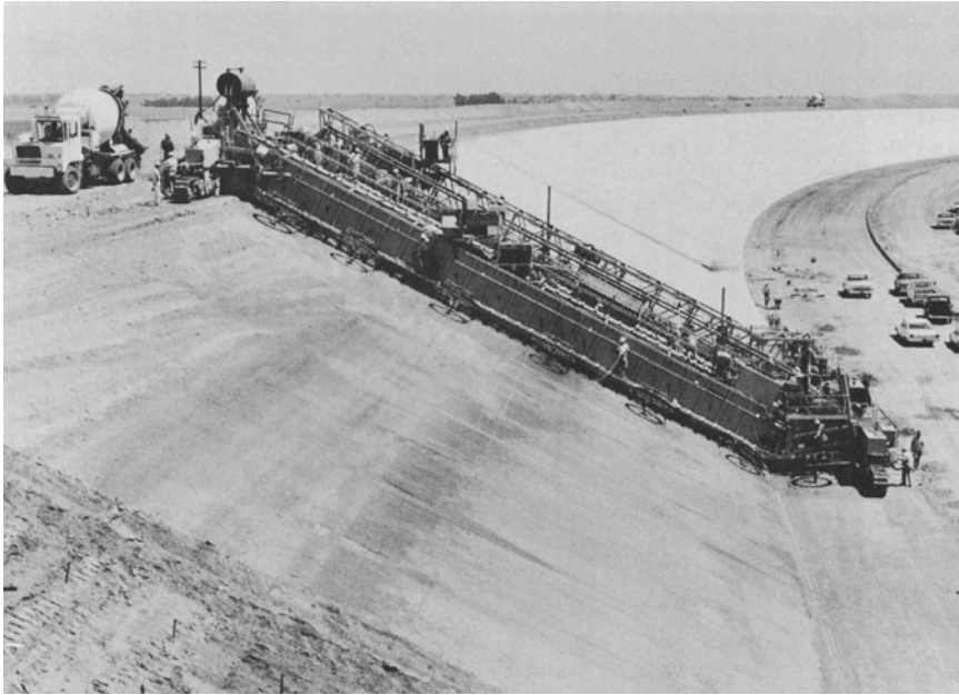
Figure 1-2 California aqueduct construction. (Photograph courtesy of the State of California, Department of Water Resources.)
