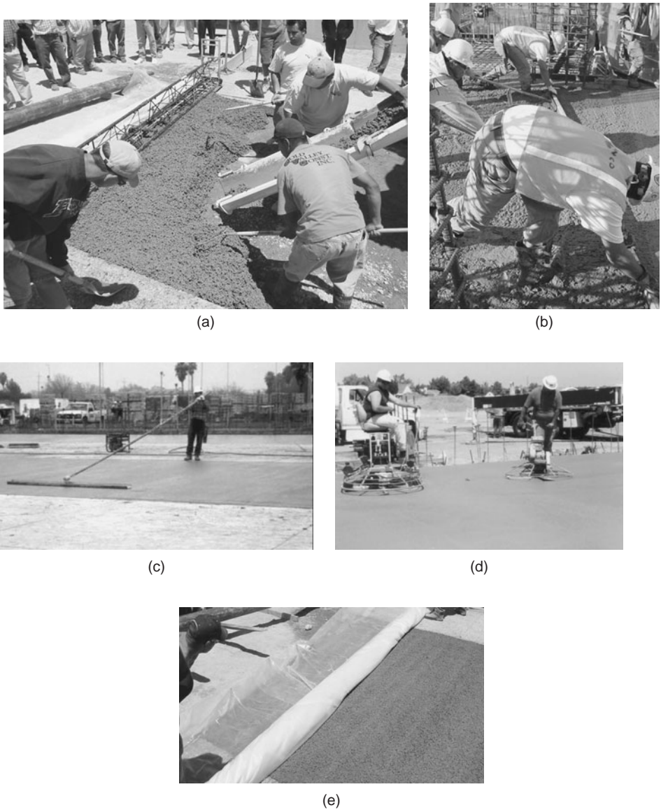
Figure 10-4 Placement and finishing of concrete slabs. (a) Delivery of the concrete; (b) screeding of the concrete; (c) bull floating for the removal of any high and low spots must be completed before any excess bleed water accumulates on the surface; (d) when the bleed-water sheen has evaporated and the concrete sustains foot pressure with only slight indentation, the surface is ready for floating and final finishing operations; (e) application of polyethylene sheet on the concrete surface to prevent moisture loss.
