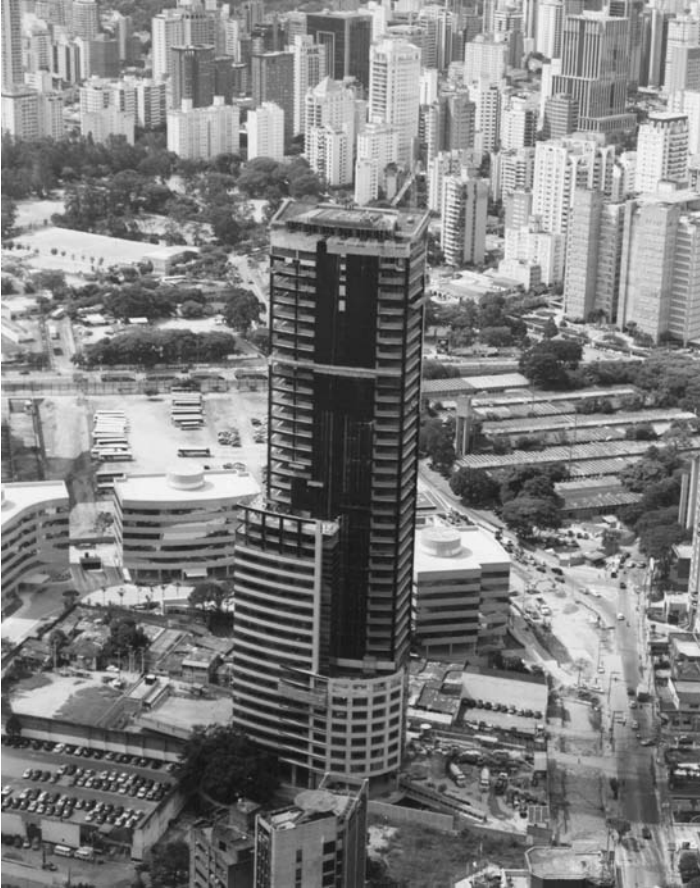
Figure 12-4 Construction of the e-Tower building in São Paulo, Brazil. (Courtesy of Helene, P., and Hartmann, C, HPCC in Brazilian Office Tower, Concr. Int. , Vol. 25, No. 12, pp. 64–68, Dec. 2003.)
