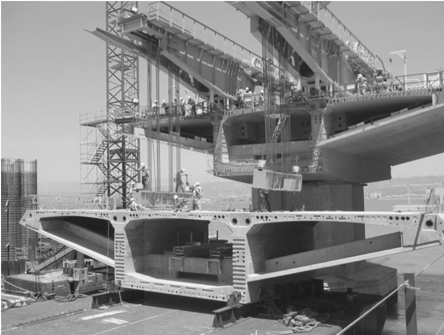
Figure 1-9 Precast concrete girders under installation for the Skyway Segment of the eastern span crossing the San Francisco Bay. (Photograph courtesy of Joseph A. Blum.)
