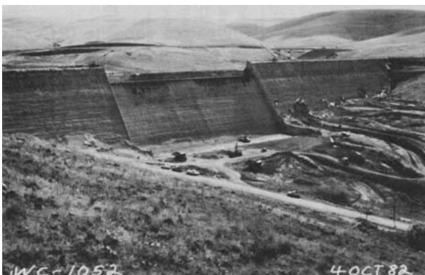
Figure 12-29 Willow Creek Dam, Oregon, the world's first all-roller-compacted concrete structure, shown about 18 weeks after the start of placement. (Photograph courtesy of Schrader, E., Concr. Int. , Vol. 6, No. 5, 1984.)
