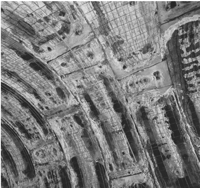
Figure 5-13 Fire damage to the concrete lining of the Channel Tunnel. [Photograph courtesy of Paul Acker]
