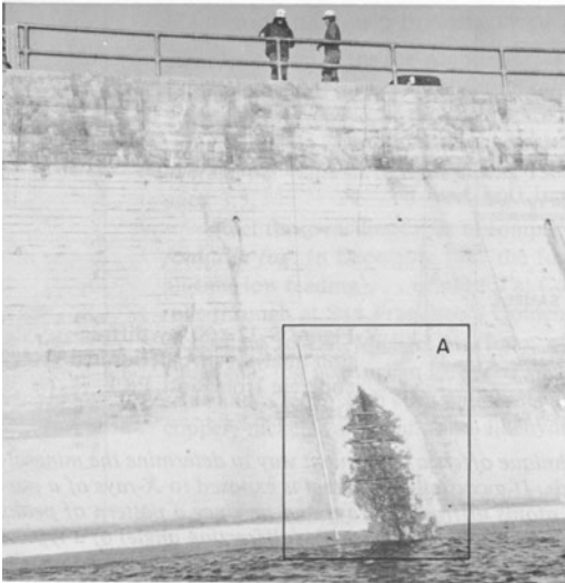
Figure 5-17 Sulfate attack on concrete in Fort Peck Dam, 1971. (Photographs courtesy of T.J. Reading, formerly Materials Engineer of the Missouri River Division, U.S. Corps of Engineers.)
