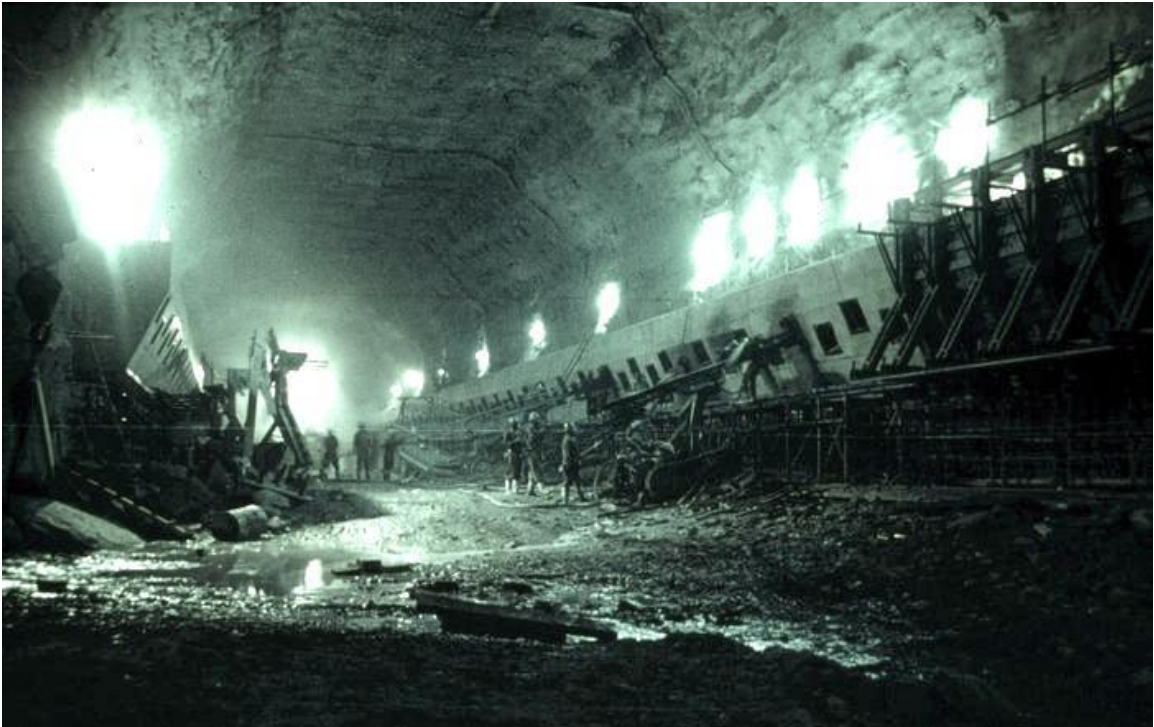
Figure 26: Cast in place concrete crane beam being anchored to the sidewall of the power cavern of the Drakensberg Pumped Storage Project in South Africa.
