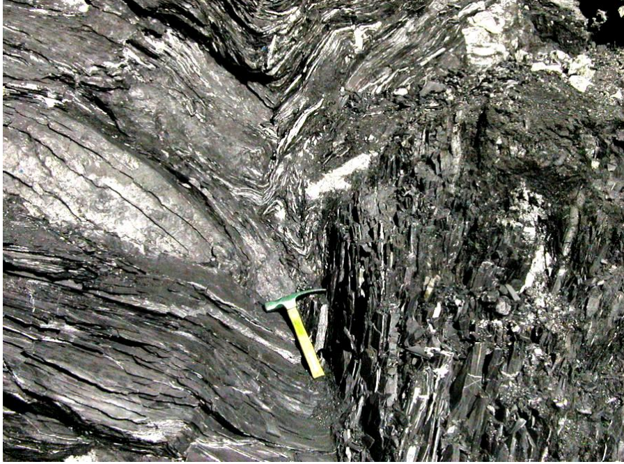
Figure 3: Tectonically deformed and sheared graphitic phyllite in the face of the Yacambú-Quibor tunnel at a depth of 1200 m below surface.
