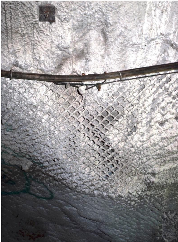
Figure 7: Chainlink mesh, while very strong and flexible, is not ideal for shotcrete application because it is difficult for the shotcrete to penetrate the mesh.
