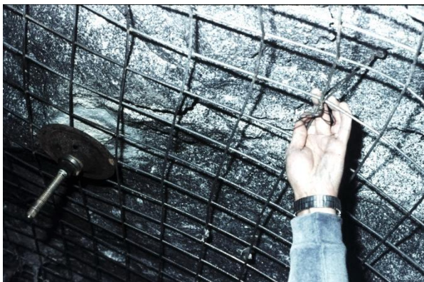
Figure 8: Welded wire mesh, firmly attached to the rock surface, provides excellent reinforcement for shotcrete.
