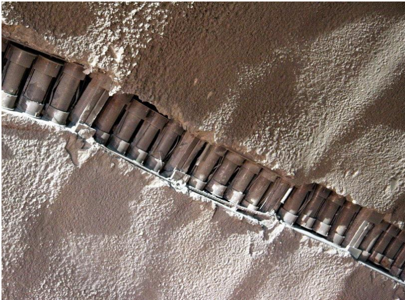
Figure 17: A row of stress controllers installed in a slot in the shotcrete lining in a tunnel
