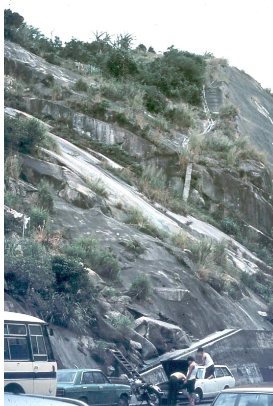
Figure 4: The failure surface defined by a sheet joint surface on which a small slide occurred during blasting of the original cut slope for the Sau Mau Ping Road. The potentially unstable slope under consideration is visible in the background.
